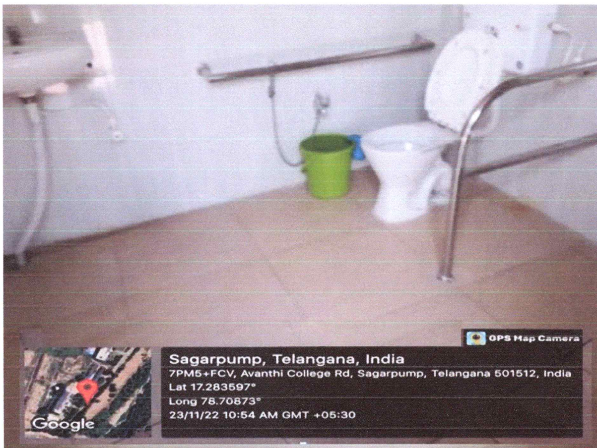
DIFFERENTLY ABLED FRIENDLY RESTROOM
